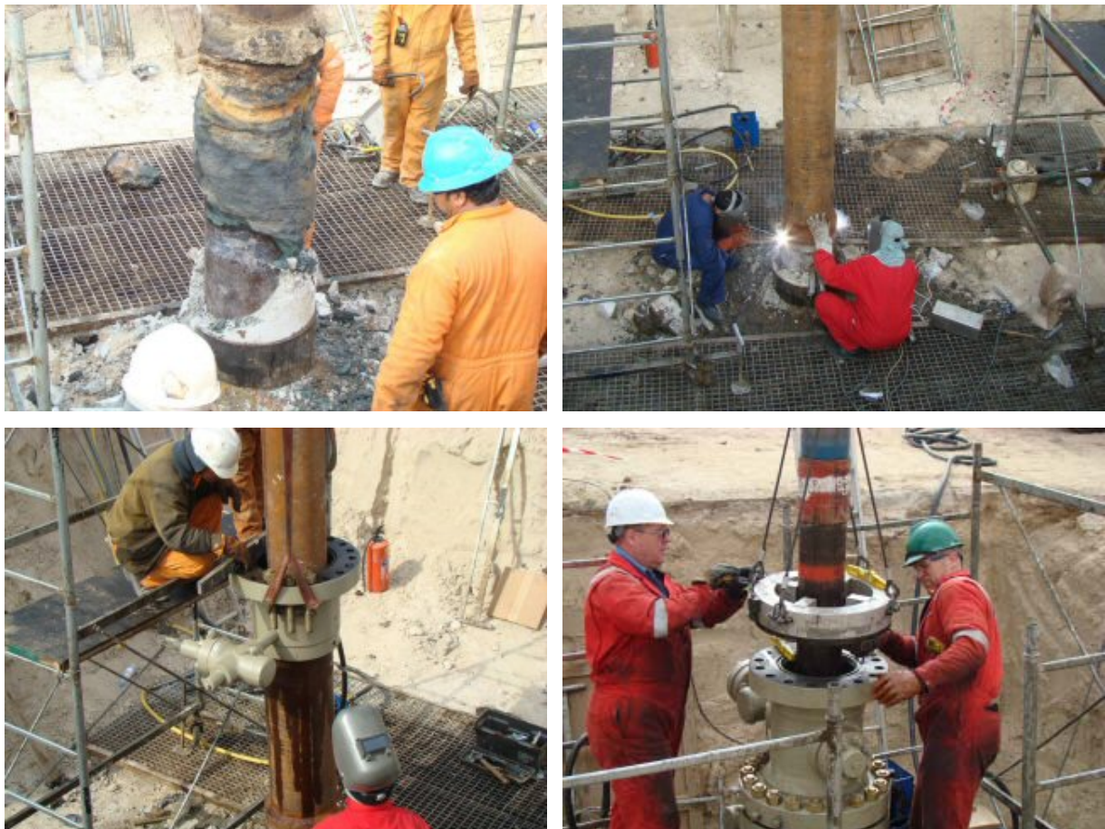
Figure 2: Casing cutting and repositioning of a wellhead after a leak path was identified
